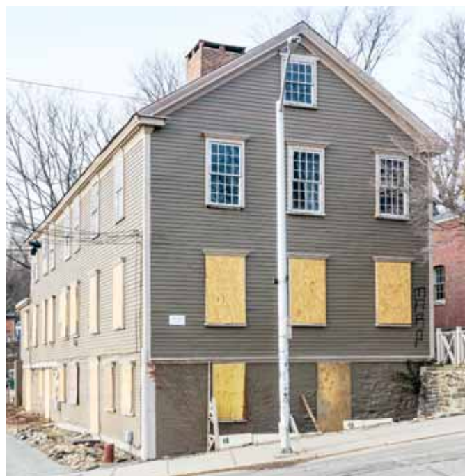
The 1785 Welcome Arnold House at 21 Planet Street. Visit ppsri.org/WelcomeArnold to get involved.
